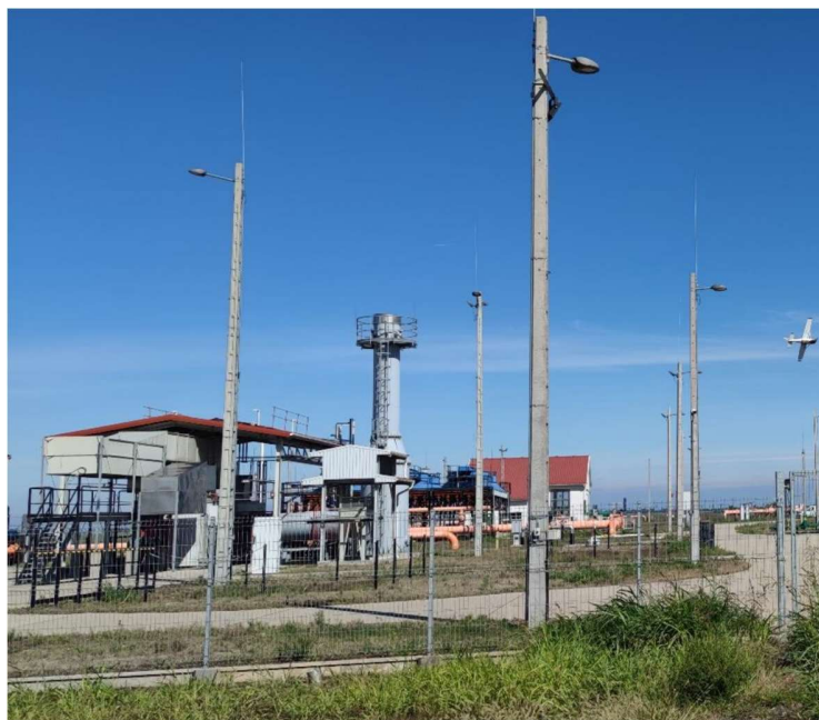
Gas turbine driven compressor units at the station
